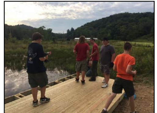
Danny Verna (center) works with fellow scouts from troop 375 on the observation platform.
