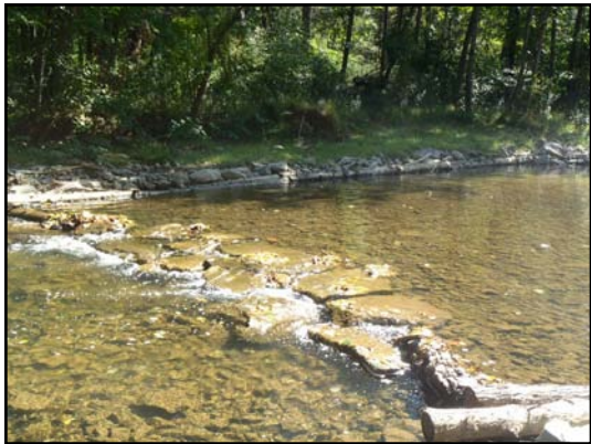
This log-framed cross vane with rock throat was installed to help narrow the channel and increase stream flow and oxygen in the water.
