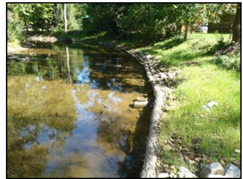
A modified mudsill will help stabilize a once-eroding bank while creating habitat for fish.
